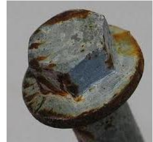
Corrosion, scale, oxide layer
